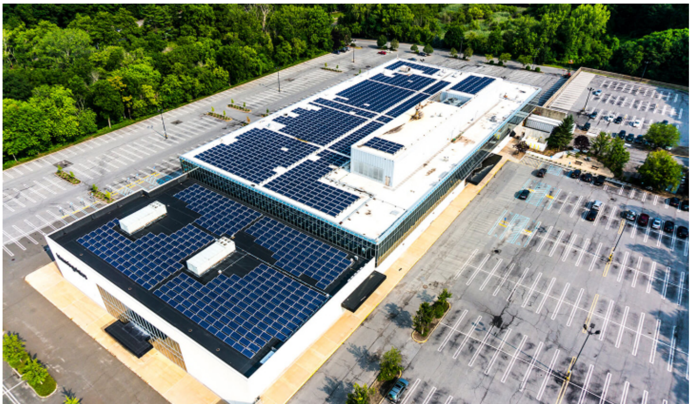
Bloomingdales Rooftop Solar System in White Plains, Source: Solar Landscape
