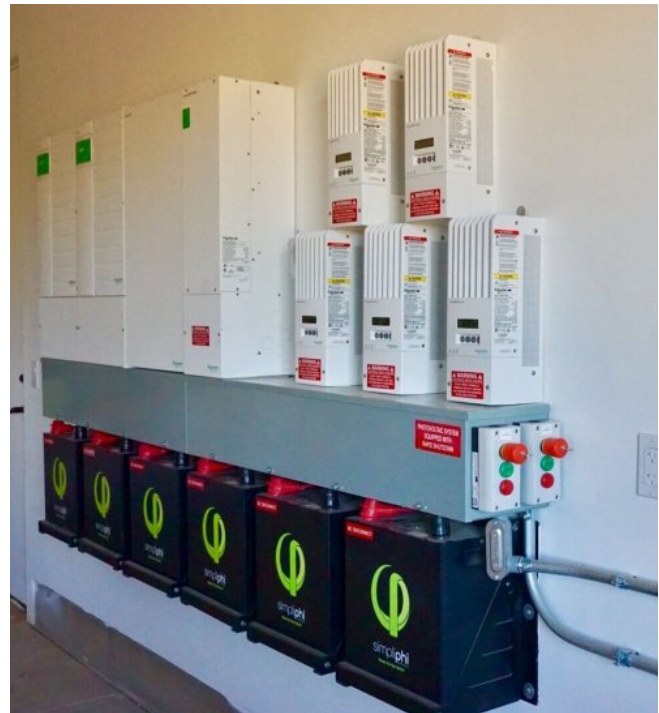
Battery System Paired with Residential Rooftop Solar
