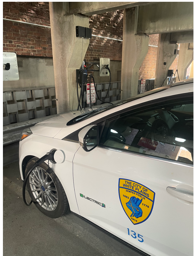
Electric Vehicle (EV) Chargers at the Lyon Place Municipal Garage and Main-Hamilton Garage
